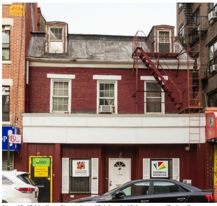
Nos. 45-47 Madison Street. Late 18th/ early 19th century. (Federal). Photo: Bruce Monroe
