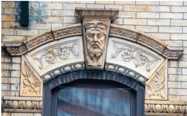
Façade details. No. 45 St. James Place (No. 22 James Street), 1884. Photos: Bruce Monroe
